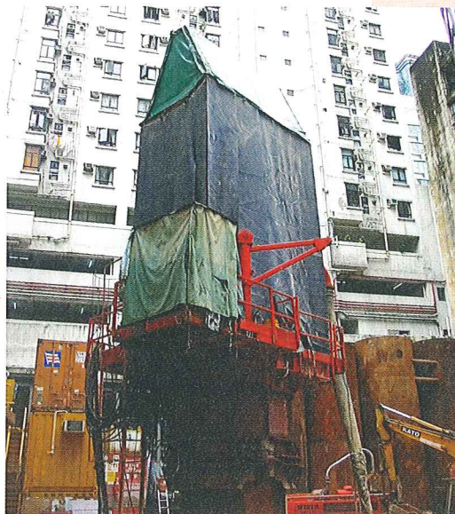
Noise enclosure for mitigating noise generated by reverse circulation drill operation 裝置隔音設備以減低因操作反循環系統鑽孔機時所產生之噪音
