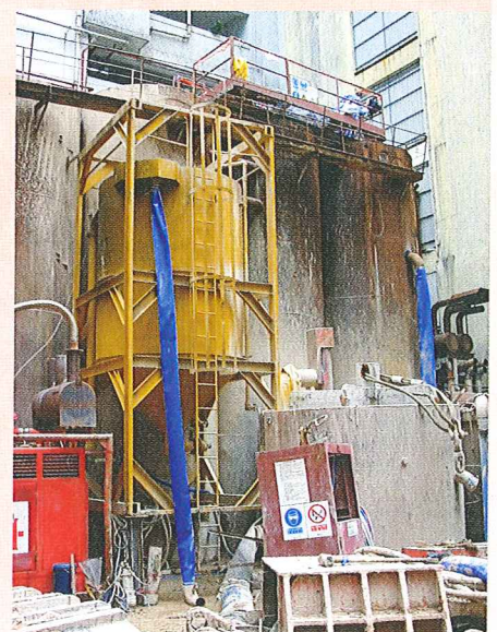
Water desliting and recycling system for bored piling works 為進行鑽孔樁工程而裝置的水質過濾及循環再用系統
