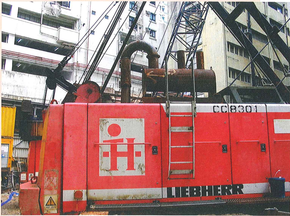
Water scrubber installed on a crawler crane to mitigate exhaust fume 吊機內安裝水性隔氣鼓以減少排出廢氣
