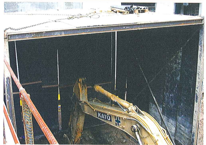
Noise enclosure for a backhoe with hydraulic breaker 裝置隔音設備以減低配上油壓式破碎機之挖泥機於操作時產生之噪音
